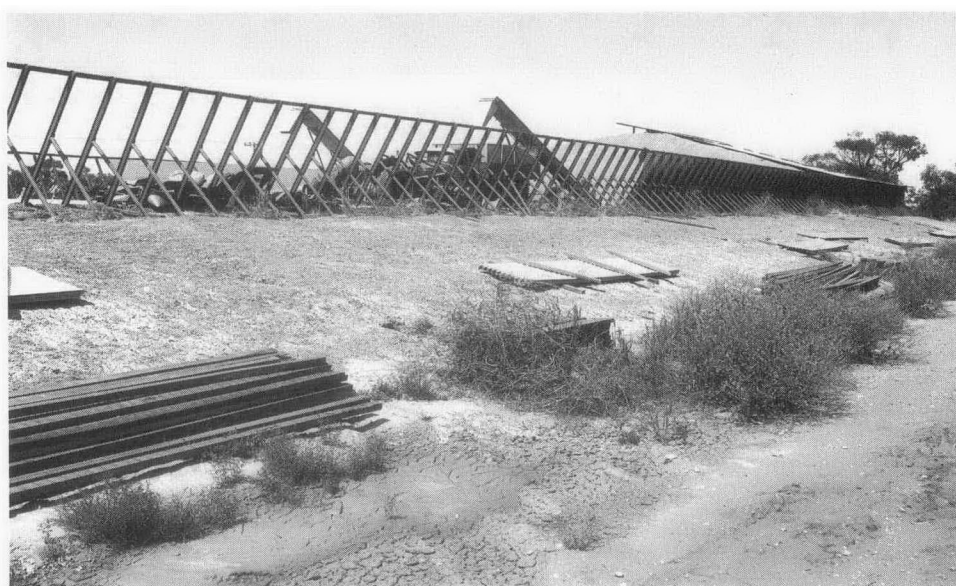
Fig. 2. (Top) 'A' frame temporary storage being emptied—note A frames and roof on grain bulk. (Bottom) 'A' frame temporary storage being emptied showing sections of roofing and side walls removed.
